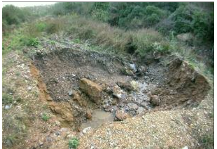
Flood damage to the stream bank of the landfill site
